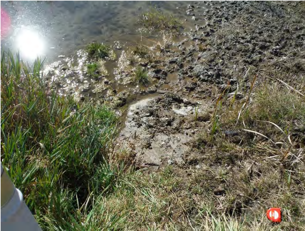
Photo 8 – Exposed liner at the south end of the west perimeter swale, adjacent to the first leachate drain outfall. Heavy deer traffic in this area could potentially penetrate the liner.
