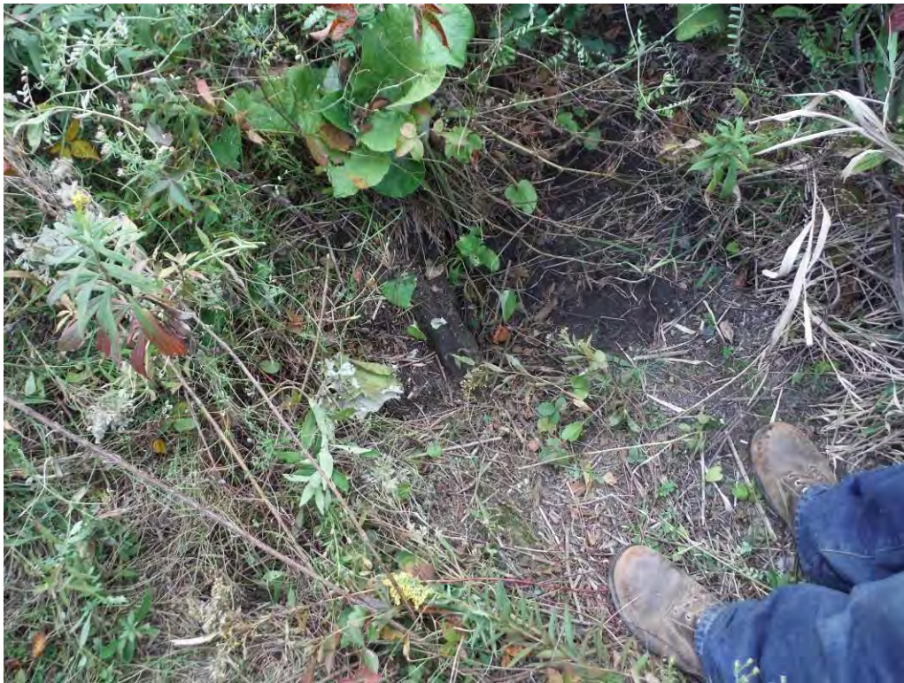
Photo 7 – Exposed geotextile and liner at woodchuck burrows near the northwest toe of the Landfill.
