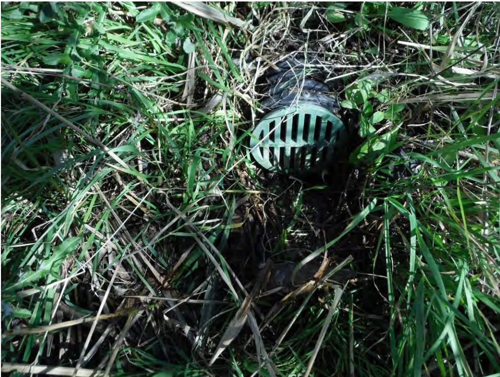
Photo 11 – Leachate Drain No. 7 outfall with animal guard.
