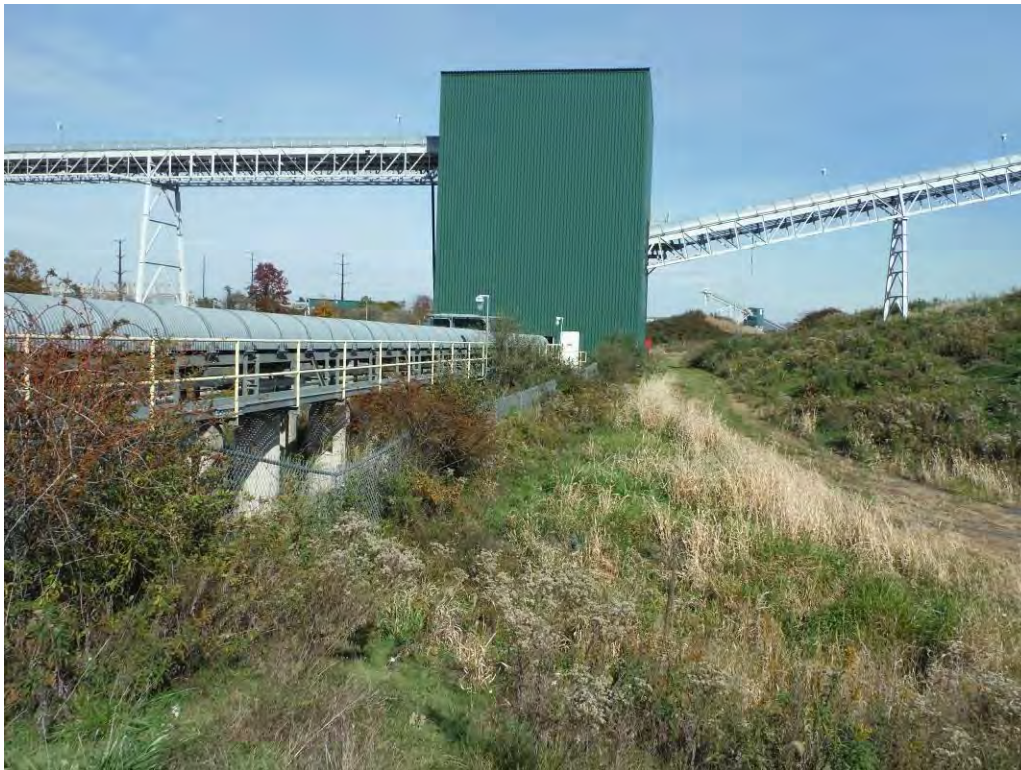
Photo 6 – Toe of the Landfill at the northwest corner, looking east. Several woodchuck holes were observed in the tall grass adjacent to the chainlink fence, which appeared to have exposed the edge of the liner. The dirty water swale at the north end is located to the left (north) of the chain link fence and may be beyond the limits of the liner.
