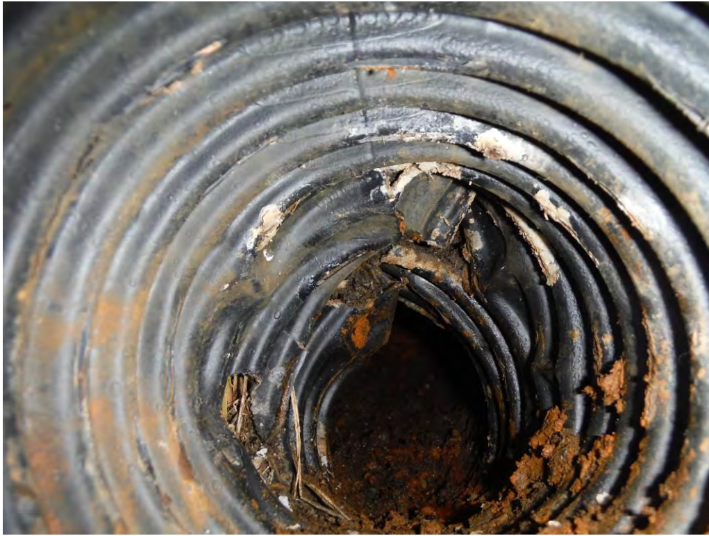
Photo 12 – Damage and plugging of the outfall of Leachate Drain No. 4.
