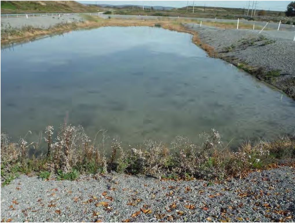
Photo 16 – Depressions in the clay liner of the leachate runoff basin.
