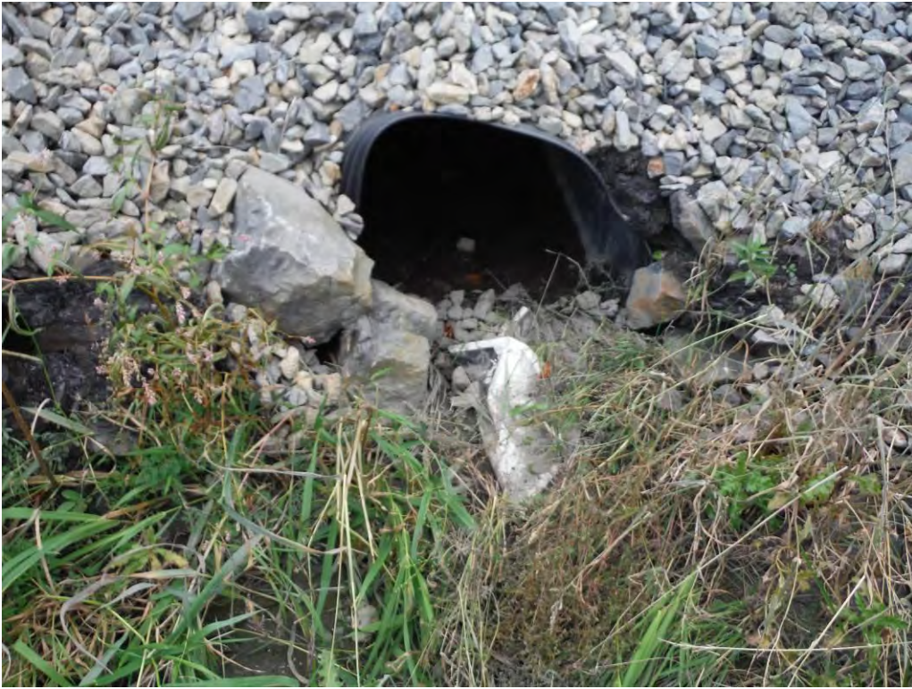
Photo 10 – Obstructed culvert passing under the conveyor building.
