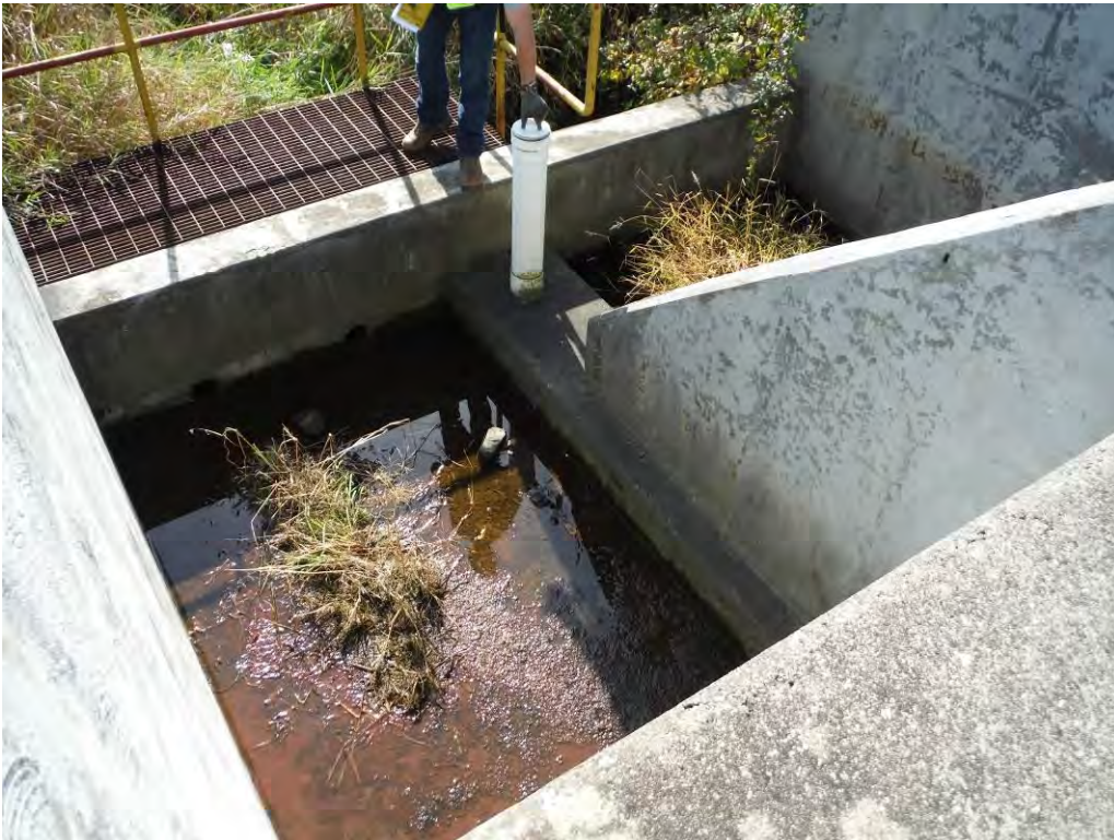
Photo 17 – Groundwater underdrain riser pipe, visible from the stream diversion outfall structure.
