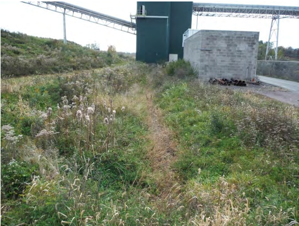
Photo 5 – North end of Cell B. The conveyor building, constructed after the Landfill, straddles the north dirty water perimeter swale.
