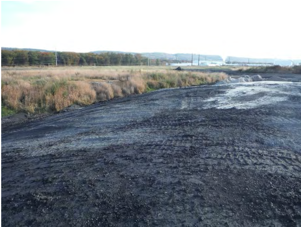
Photo 13 – Working Landfill surface showing shaped, compacted fill, dust-protection caking agent, and temporary grass cover beyond.
