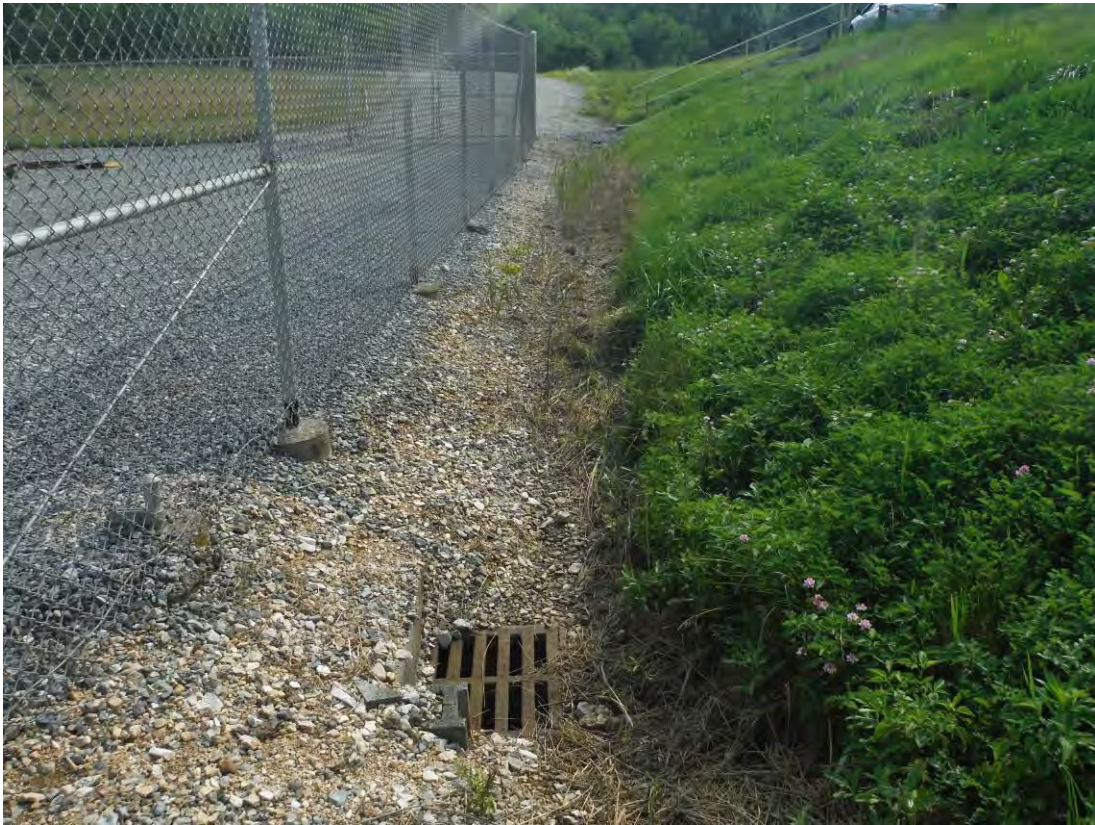
Photo 32 – Catch basin and ditch at the median dike, which has grown in and should be maintained.
