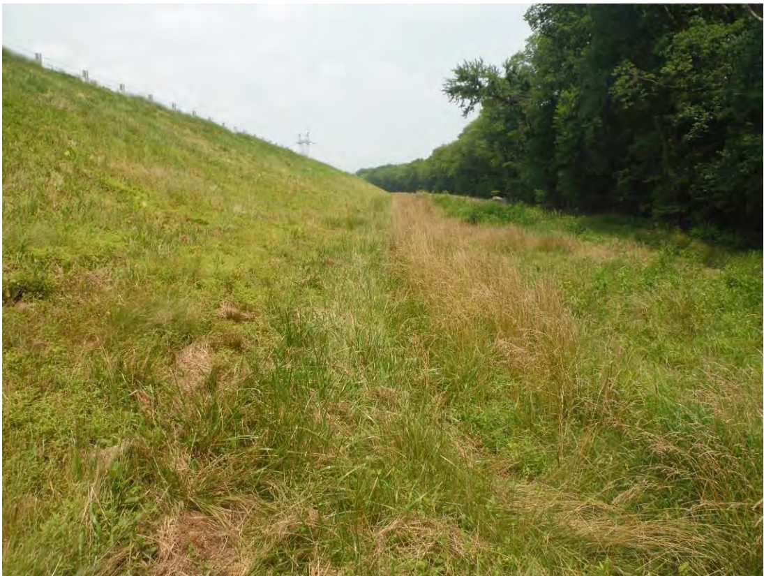
Photo 3 – Looking north at a wet area at the toe of the east embankment at about Station 1+50. Wet soils extended about 3 feet vertically up the slope.
