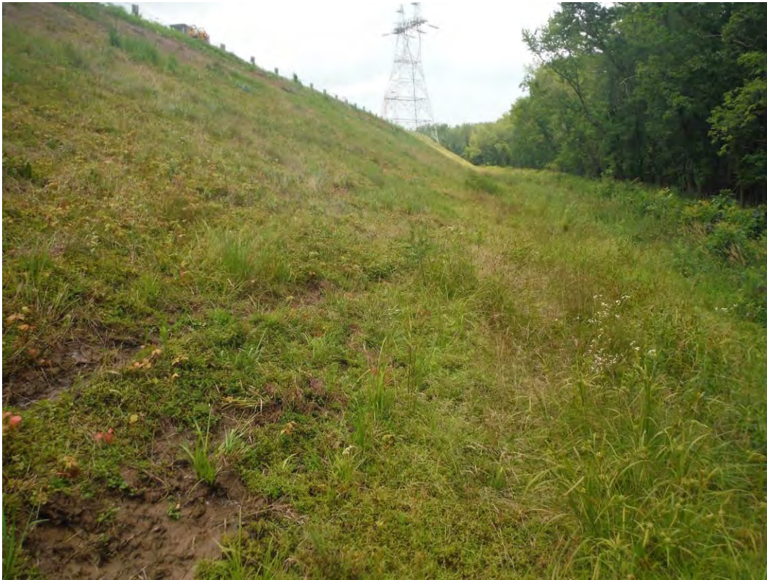
Photo 4 – Toe of the east embankment at about Station 16+00. Wet soil extended up to 8 feet vertically up the slope between Stations 16+80 and 17+60.
