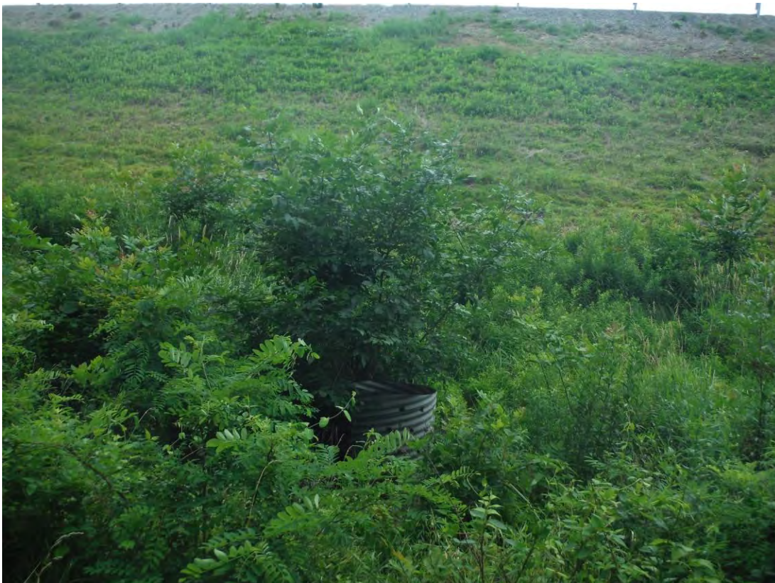
Photo 5 – Abandoned drainage structure in the ditch at the toe of the east embankment at about Station 16+00.
