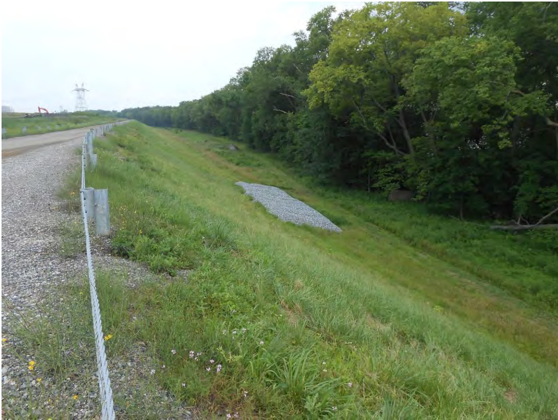
Photo 2 – Downstream slope of the east embankment, looking north from the south end, south of Station 0+00. A seepage blanket, shown in the middle of the photo, has been installed at the toe of the slope, which has historically been wet.
