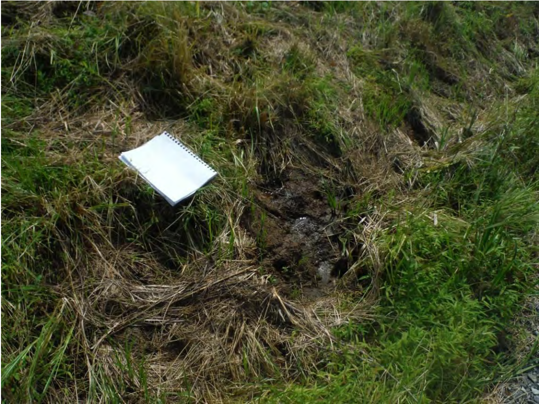
Photo 22 – Standing water in ruts at the toe of the slope at the north end of the west embankment.
