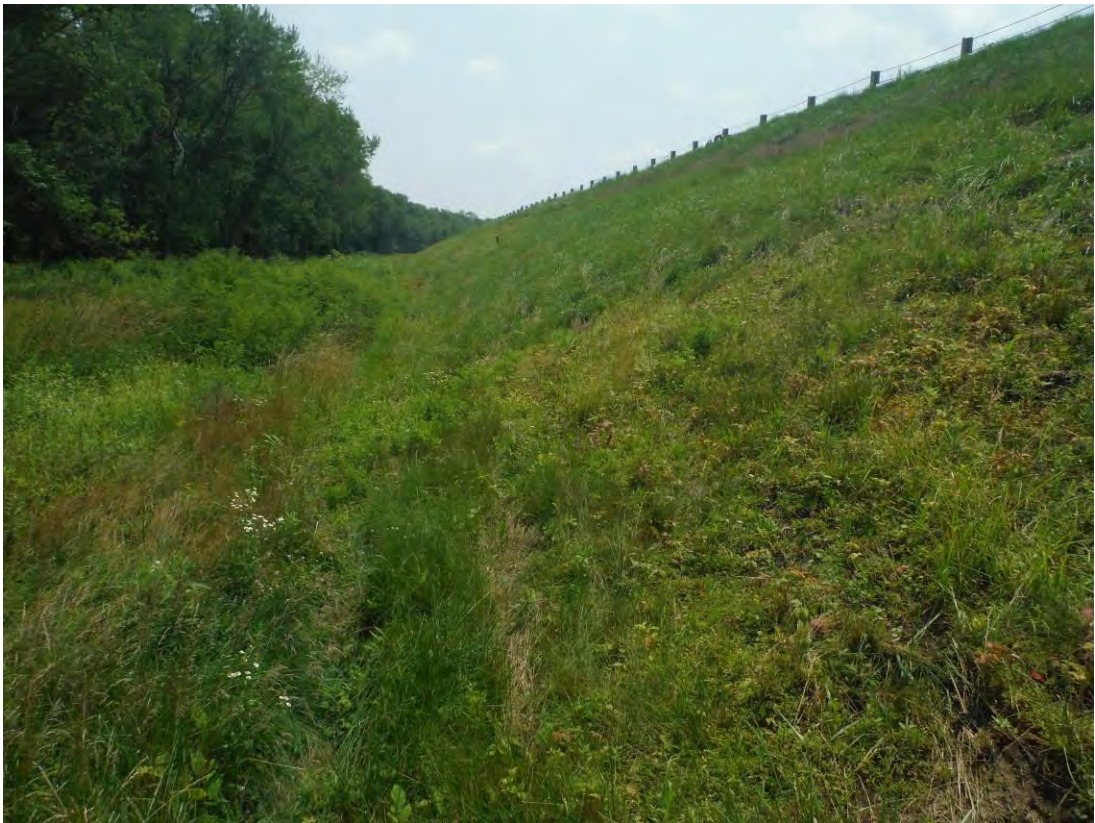
Photo 7 – East embankment looking south from about Station 24+00 at an area where previous sloughs had been repaired and re-vegetated.
