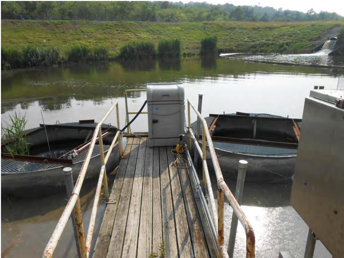
Photo 34 – The discharge structure for the polishing pond.
