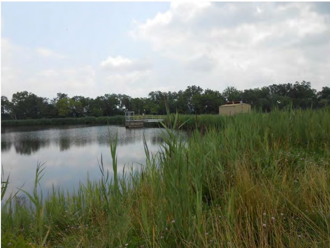
Photo 29 – Outlet structure between basin and polishing pond.
