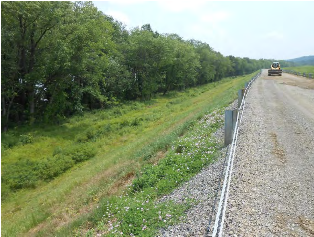
Photo 8 – East embankment looking south from about Station 23+50, showing repairs of previous sloughing on the downstream slope and the recently raised gravel crest.
