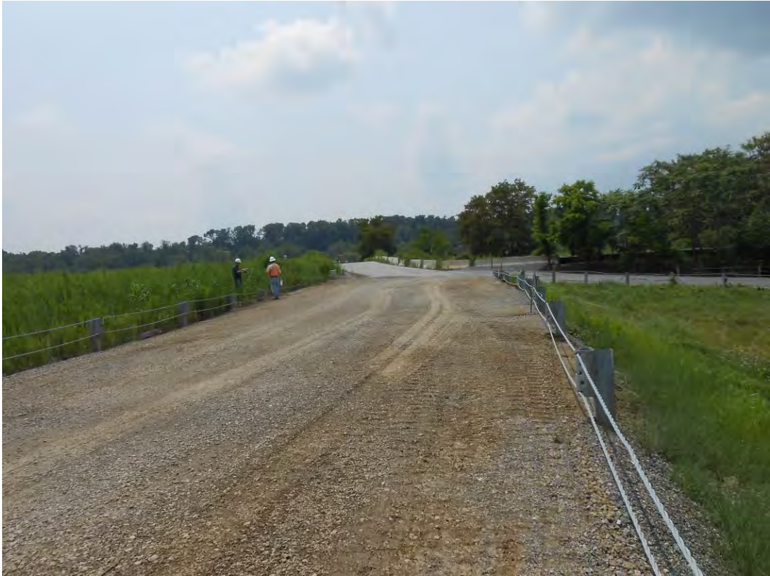
Photo 10 – Crest of the north embankment at the northeast corner of the basin. The crest was raised to the design elevation of 290 feet in 2014.
