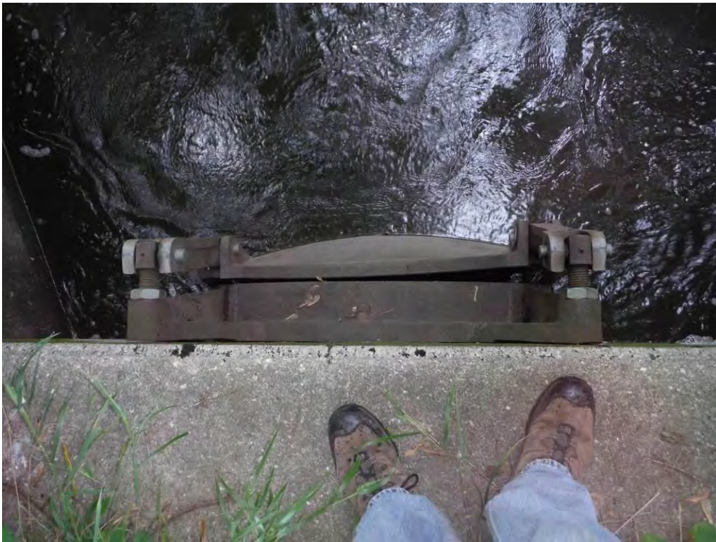
Photo 35 – Flapper valve at the end of the polishing pond discharge line.
