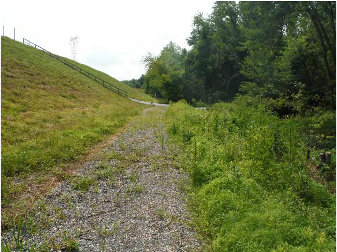
Photo 23 – Access road and grading for Monitoring Well No. 6 at the toe of the west embankment near the north end, showing irregular ground, thick vegetation and stumps.
