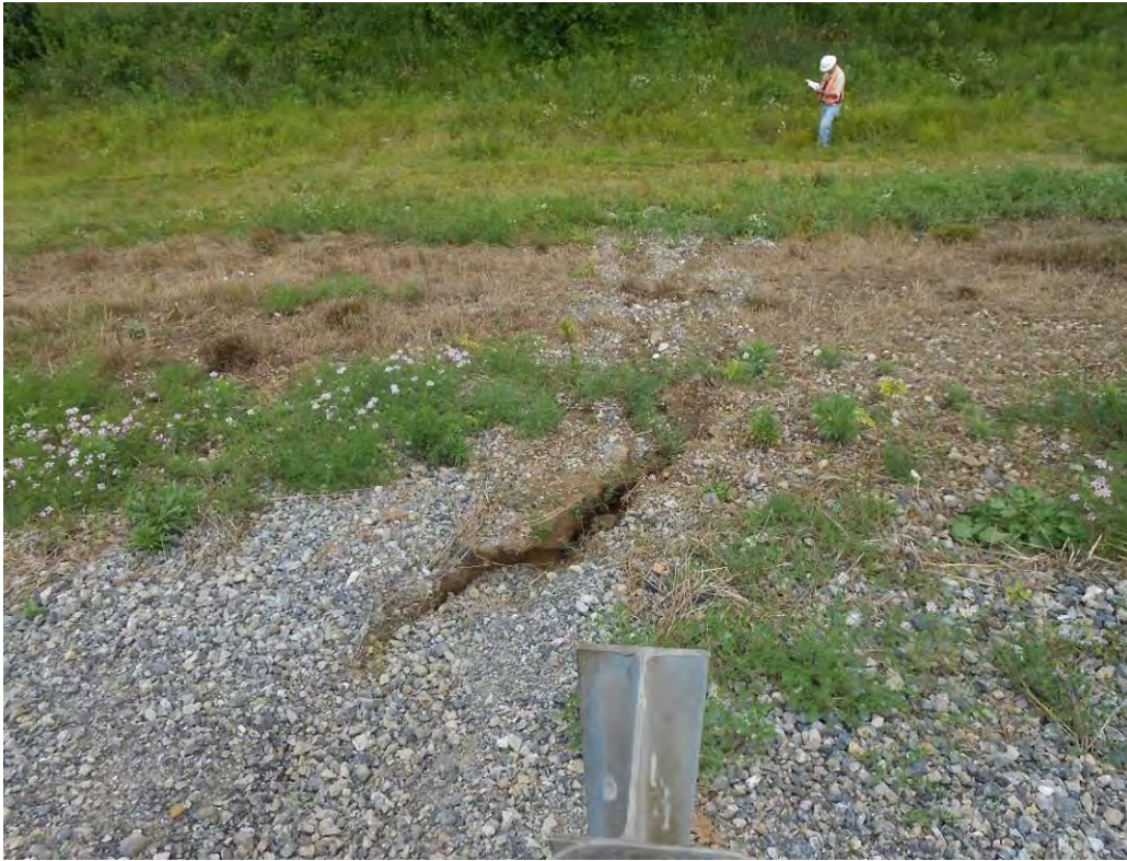
Photo 36 – Typical erosion rills observed at the top of the east and south embankments, where the crest was recently raised. This erosion rill is approximately located at STA. 18+40 on the east embankment.
