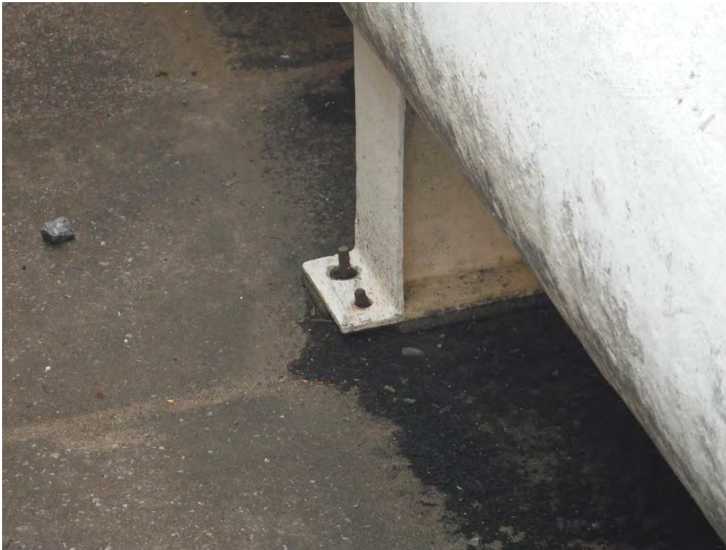
Photo 38 – Missing nuts observed on most of the bolts on the saddles of the discharge pipeline to the polishing pond.
