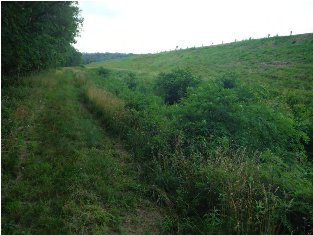
Photo 6 – East embankment looking south near Station 16+00. Heavy vegetation at toe indicates a wet area where equipment could not operate.
