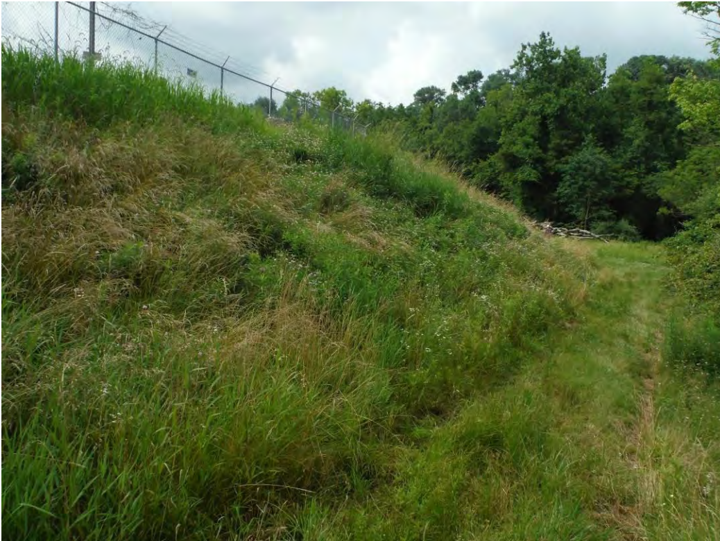
Photo 24 – Downstream slope of the west embankment near the north end, where an old slough was repaired. Grass on slope was chest high and downed trees had not been cleared.
