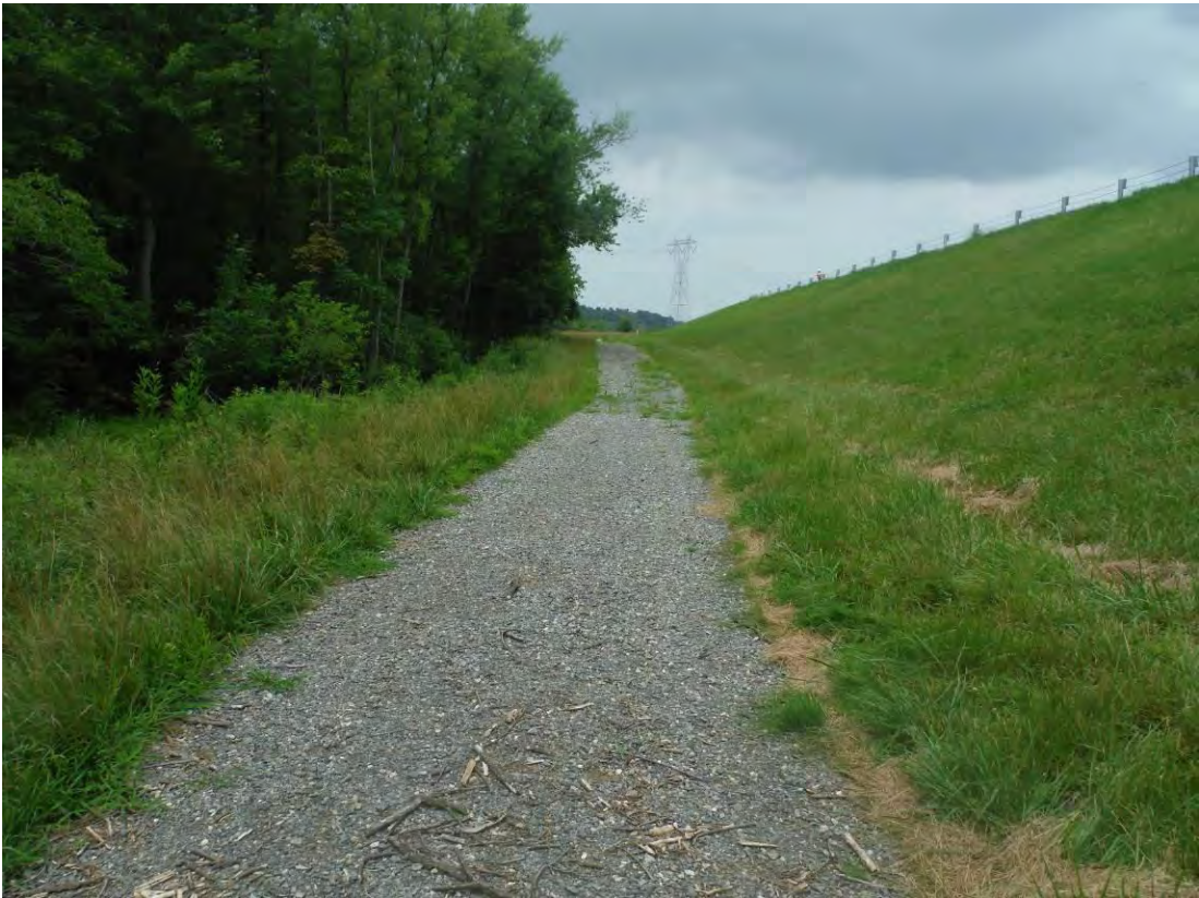
Photo 17 – Downstream slope of the west embankment, looking north from the south end. Note the new gravel access road along the toe.
