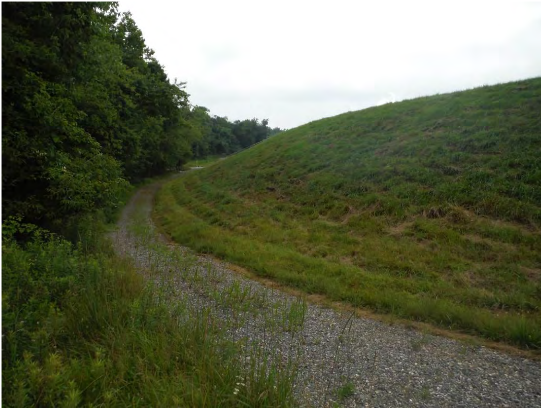
Photo 20 – Toe of the west embankment where significant disturbance was observed in 2011. The area has been regraded and reseeded. Wet soils and rutting were observed previously. A new gravel access road was installed along the toe in 2015.
