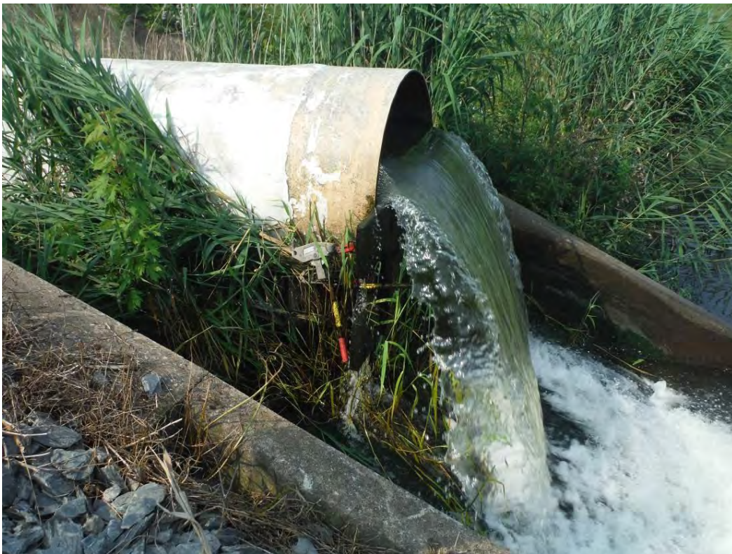
Photo 39 – Discharge pipe through the median dike observed to be 2/3 blocked with a timber exit weir. The spillway adequacy analysis assumed this discharge structure to be at full capacity. Maintenance staff were aware that the weir needs to be removed during a flood.
