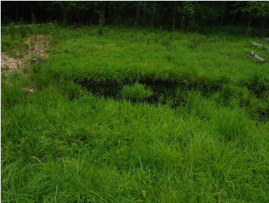
Photo 14 – Pool of stagnant standing water at the toe of the downstream slope of the polishing pond.
