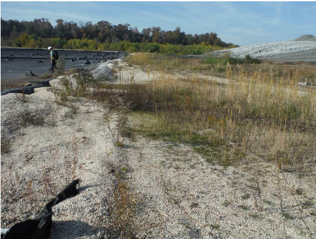
Photo 9 – Irregularly formed section of the separation dike between the active and inactive parts of Cell 1. This section of the dike should be reformed with a minimum height of 4 feet, as shown on the Project drawings.
