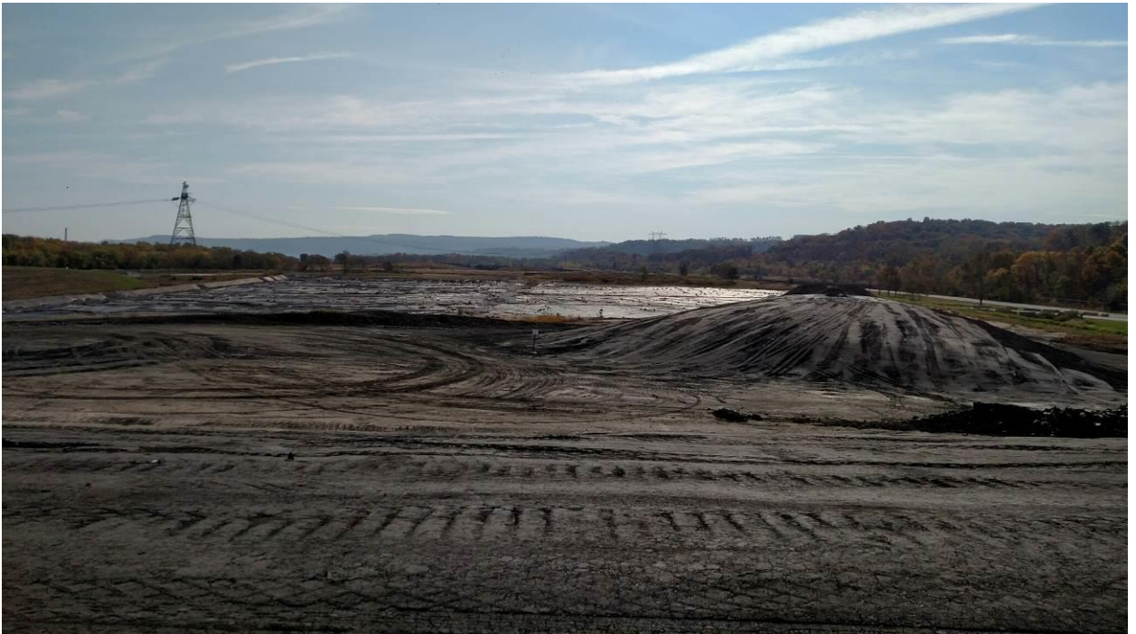
Photo 5 – Working surface of Cell 1, with the inactive part of Cell 1 in the background.
