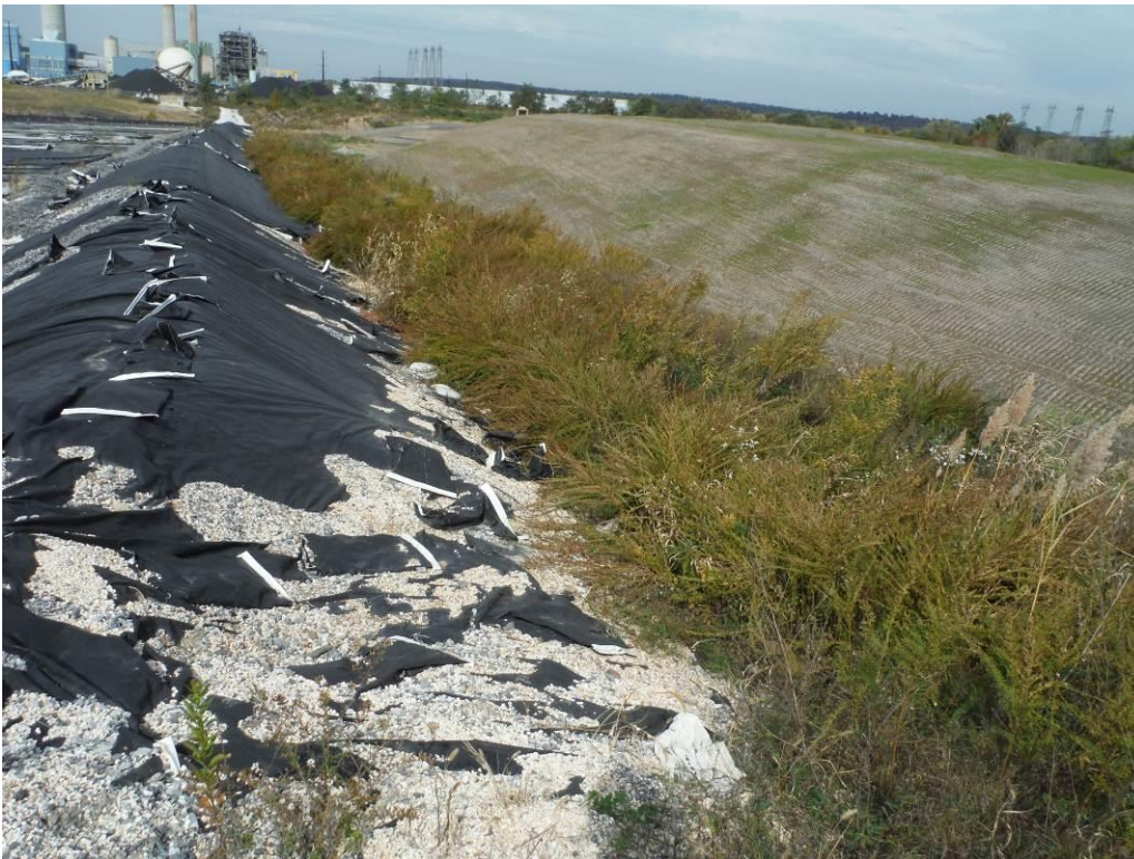
Photo 11 – Overgrown ditch along the east edge of the inactive section of Cell 1.
