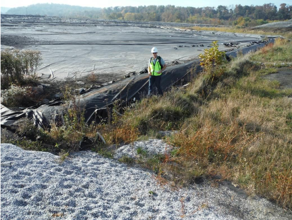
Photo 8 – Separation dike between the active and inactive parts of Cell 1, looking southwest. This section, at the southeast corner of the active part of Cell 1, is well formed, though it appeared to be less than the 4 foot height shown on the project drawings.
