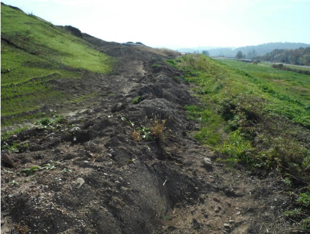
Photo 10 – Ditch at the northwest corner of Cell 1, under construction. The section to the left will convey contaminated stormwater run off to the south, and the ditch to the right conveys clean stormwater run off to the north.
