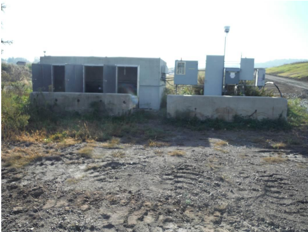
Photo 16 – Mechanical building housing the leachate collection and leakage detection sump pumps.
