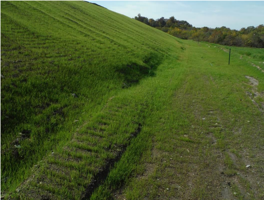
Photo 12 – Locally steep, irregular slope along the north edge of the Cell 1. Talen noted that this fill was temporary and final filling and grading would take place in the near future.
