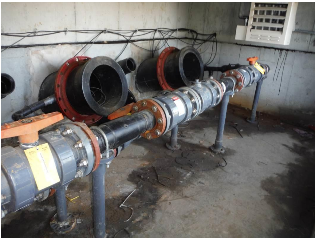
Photo 17 – Sump pumping system.
